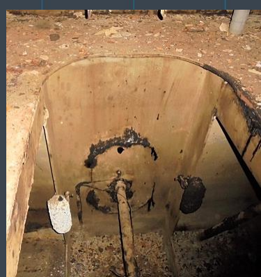
CONDITION BEFORE REPAIR
